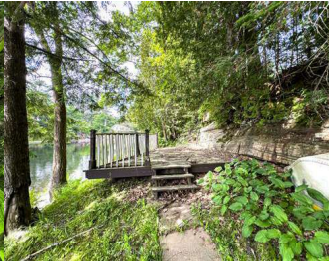
Deck at water (in need of repair)
